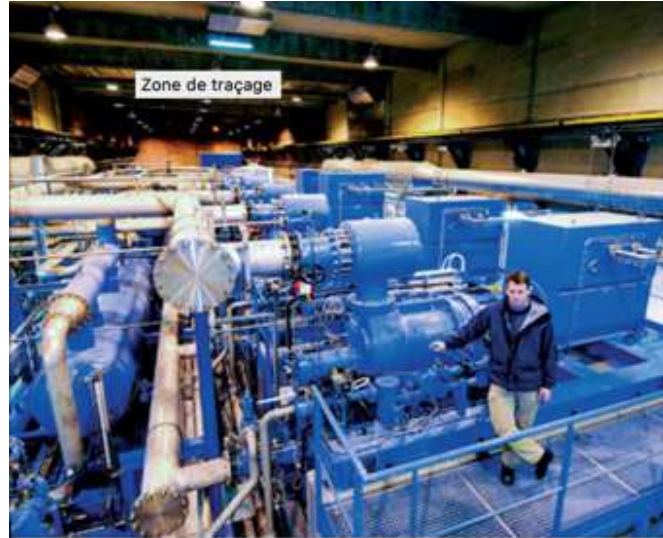
One of the 8 groups of refrigeration compressors used by the current LHC (Image: CERN)
